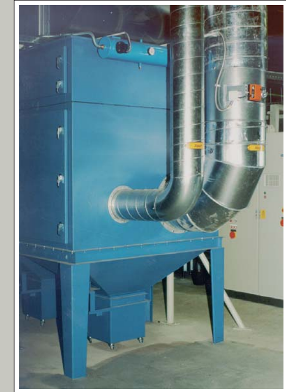
Cartridge filter – central system with a capacity of 12000 m 3 /h for welding and sharpening/grinding workplaces in train works.
