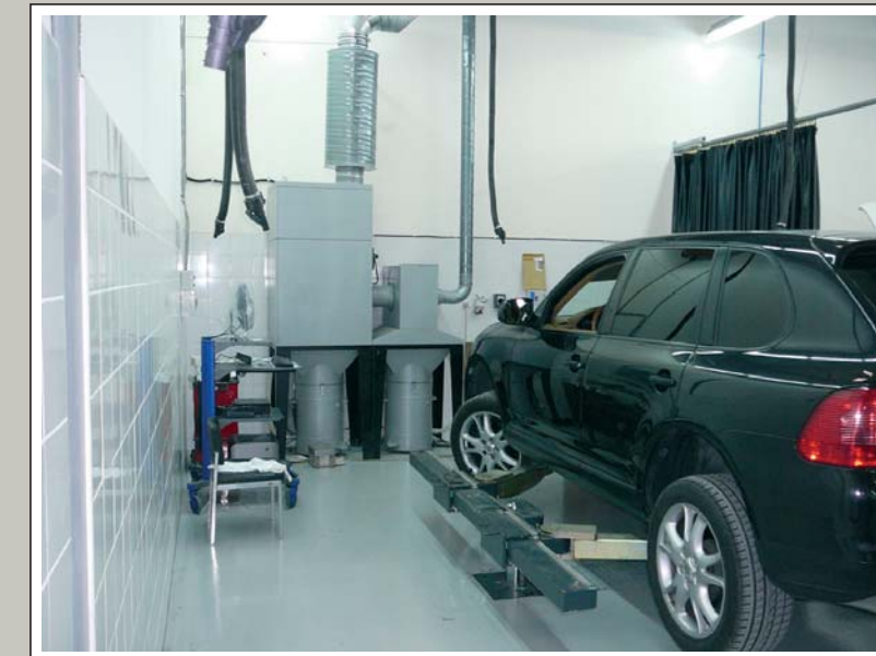
High vacuum filtering unit with spark protection monitoring (500 m 3 /h) for 2 aluminium workplaces in the body repair shop.
