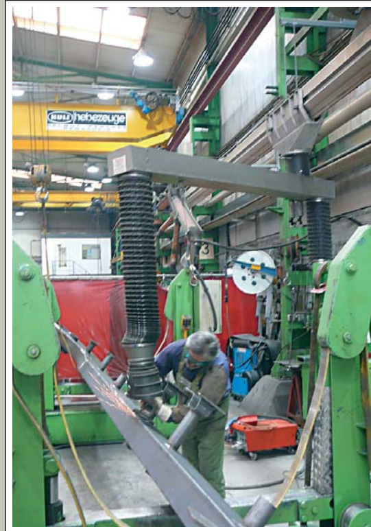
Aluminium rail system type SSK 290 with moving trolley and a extraction telescope arm for welding and grinding in a industrial workshop with long pieces.
