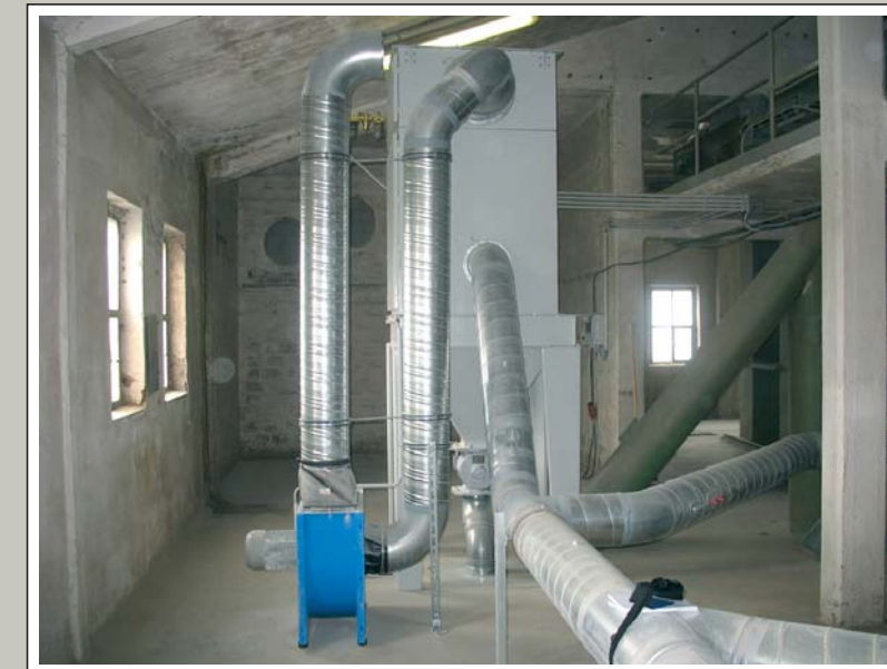
Atex-cartridge filter – central system with a capacity of 2000 m 3 /h for extraction in storage silos with worm gear discharge for medium feedback, including expansion flap.
