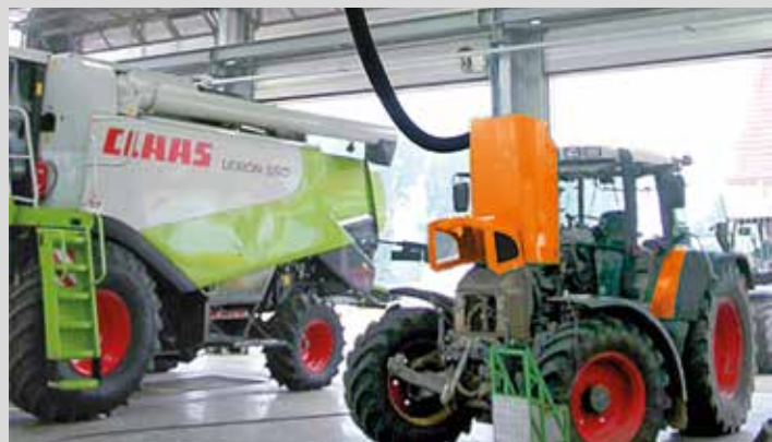
Extraction unit for overhead exhausts.
