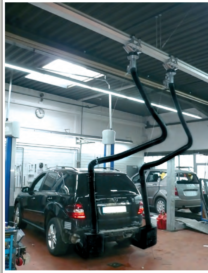
2 SLS – Car systems running in a suction rail from type SSK 150 for cars with double-flow exhaust pipes at a Mercedes-Benz workshop
