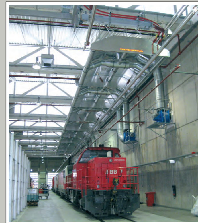
Extraction cover at ÖBB, length 40 m, with segment extraction via smoke and heat detectors during coming in and leaving of the diesel locomotive in the hangar to adhere to health protection at the workplace (analogously our TRGS 554).
