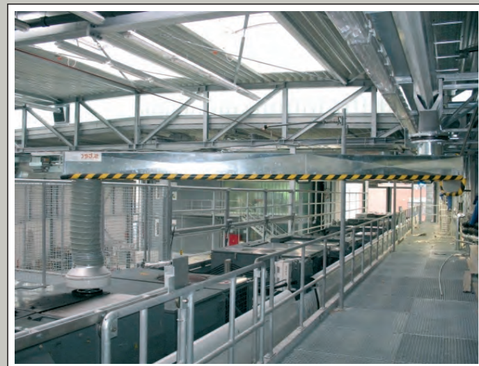
Exhaust gas extraction for diesel railcars for regional railway service with an SSK 290 rail system – 60 m length – with a cantilever arm, NW 250, length 5 m.
