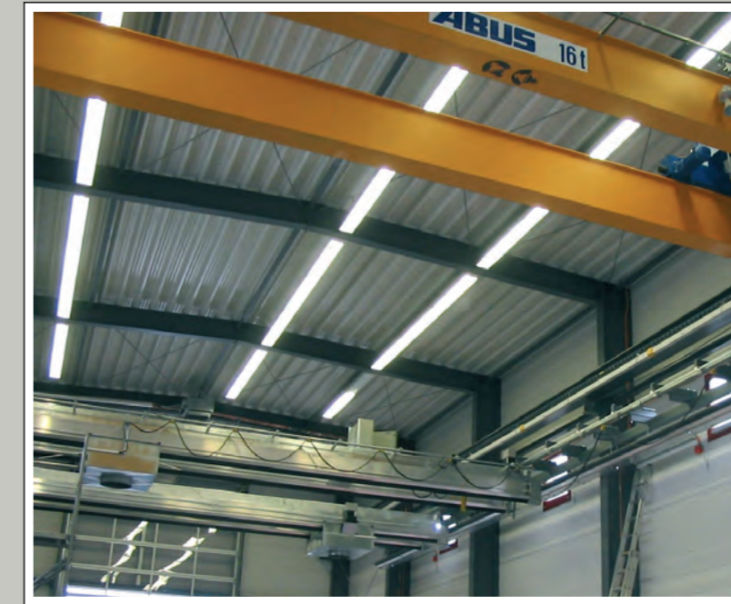
Exhaust gas extraction unit for diesel railcars and diesel locomotives in a service workshop at Westerwaldbahn with a crane-like SSK 900 rail system – 60 m long – with two SSK 900 extraction racks – 14 m width – self-supporting and movable in three axes.
