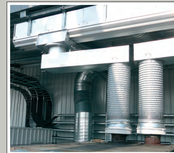
Two extraction hose carriages, NW 560, for a diesel emergency generator, 1,100 KVA, telescopic with a reach of 2.5 m, for an extraction volume of 25,000 m 3 /h.
