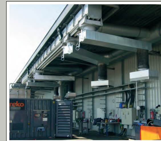
Rail system, SSK 1350, length 30 m, with four NW 560 extraction carriages for performance endurance tests on diesel operated emergency generators with up to 1,100 KVA, manually movable, pivotable and height adjustable.
