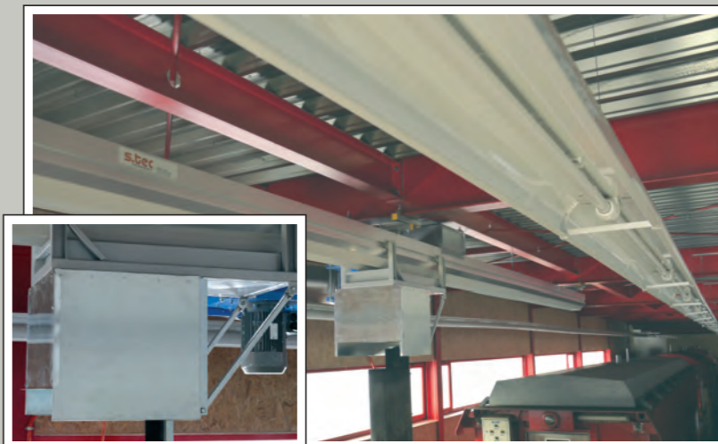
Diesel locomotive extraction, going with and automatically releasing, for the fire brigade at SBB in the St. Gotthard tunnel, with 5,000 m 3 /h, combined with a Firemaster connecting and separating device via an SSK 580 rail system.
