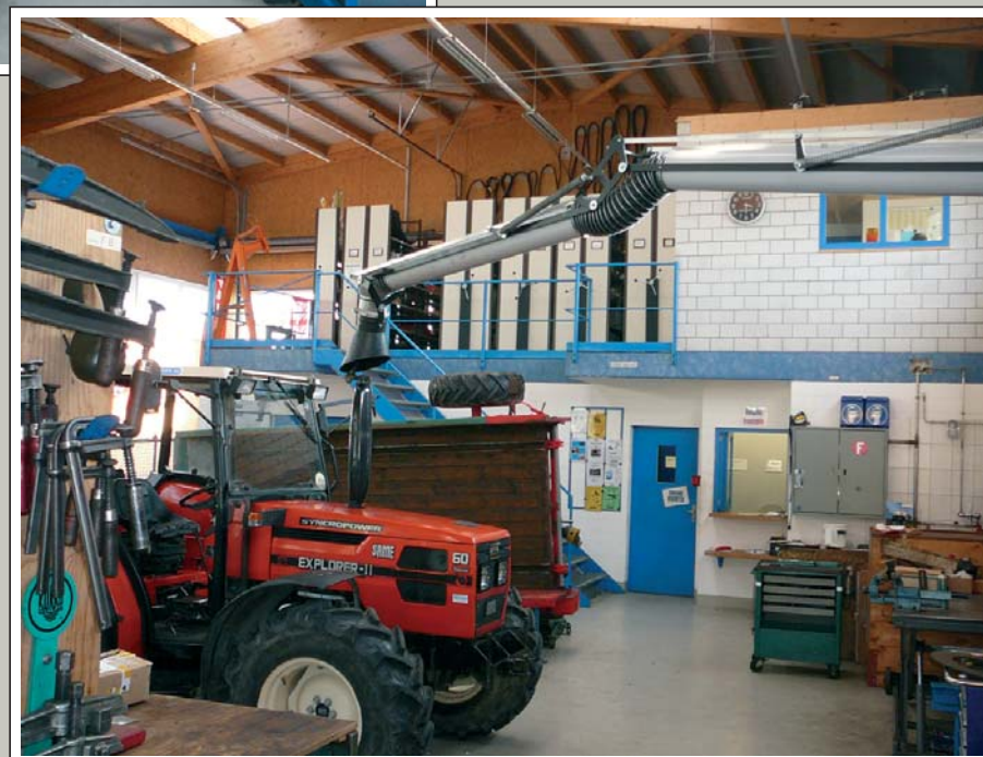
Extraction system with large reach in the agricultural machine shop
