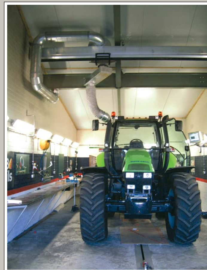
Performance rest / dyno test bed for haulers. Rail system SSK 450 with high temperature extraction unit
