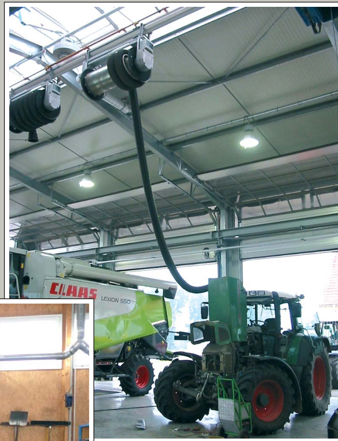
Mobile hose reel running electrically in the SSK- rail system by radio remote control.
