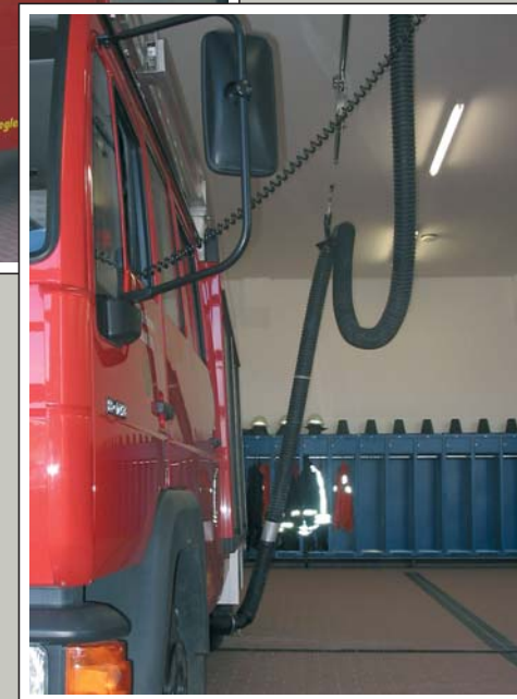
FireMaster Airpulse A sleeve operated with compressed air covers the exhaust pipe until the vehicle leaves the shop - a tried technology in automatic operation.
