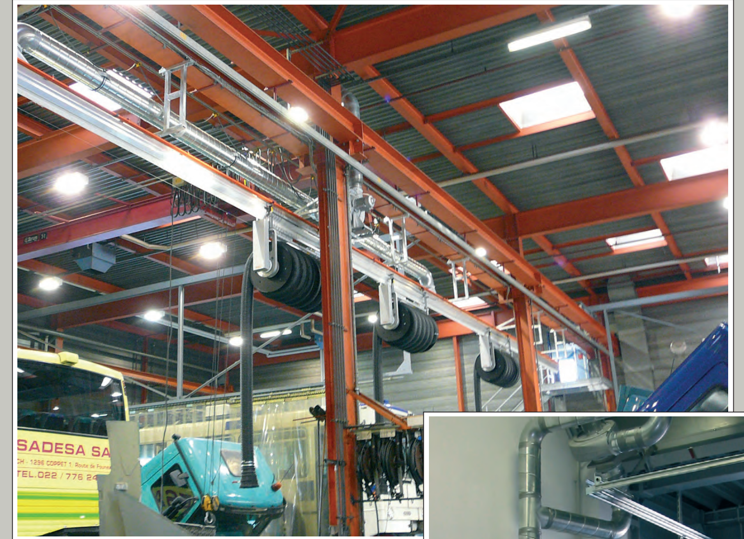
Exhaust extraction system in a Mercedes Benz truck workshop with 8x working bays in 4 rows. The workshop is partially covered by a movable crane. Exhaust extraction solution with electrical movable hose reels in a rail system from type SSK 450.
