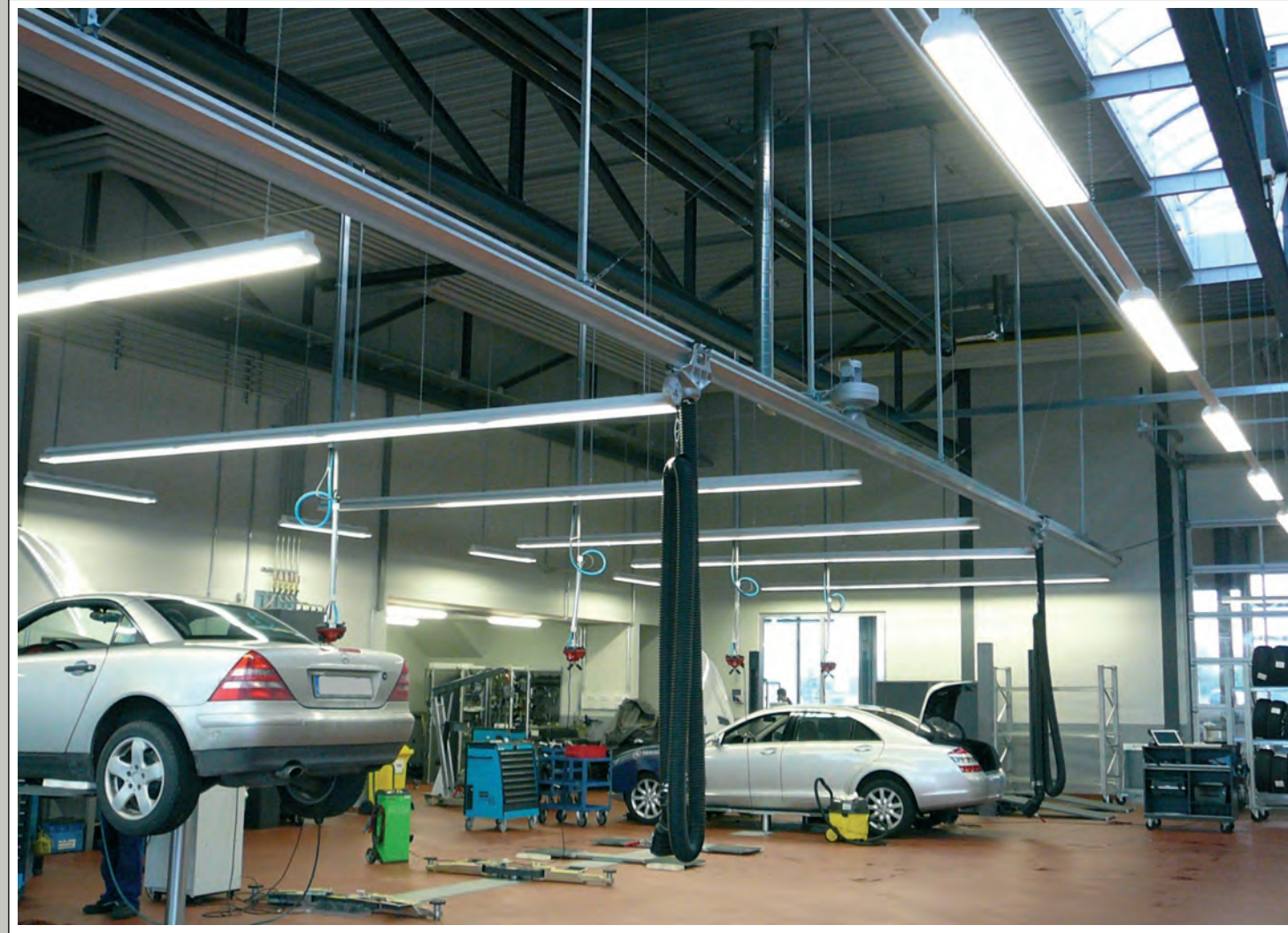
Car workshop with rail system, 2x extraction trolleys equipped with hose 5m and funnel. The exhaust extraction fan is mounted directly on the rail.
