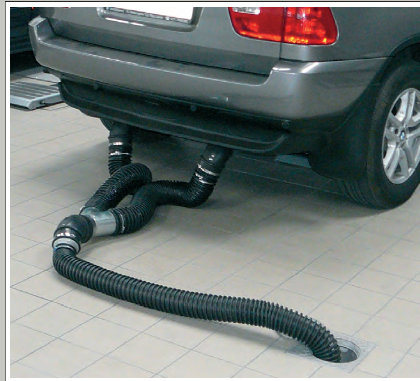
Kit suitable for underground exhaust extraction systems, serving 2x single exhaust pipes. Picture was taken in a BMW workshop with 10 working bays.
