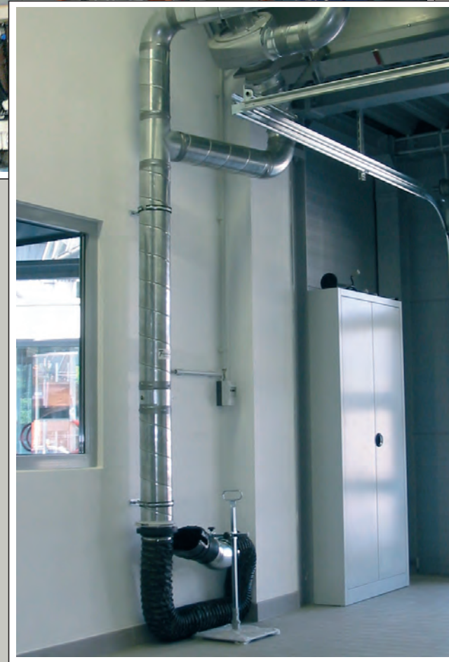
Exhaust extraction system for emission tests in a Porsche workshop. Extraction fan equipped with hose ø150 mm, and a special standing funnel. A second separate connection is available for a possible second exhaust pipe.
