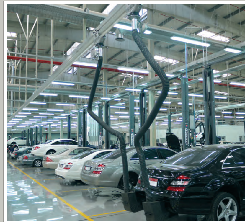
Exhaust extraction system in Mercedes Benz workshop with 240x working bays. Extraction rails equipped with the universal and exhaust pipe independent capturing element SLS.
